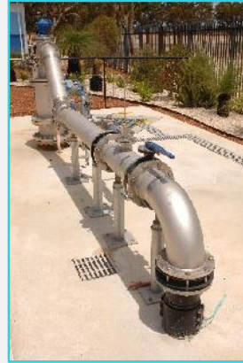
Beenyup Leederville Recharge Bore Image courtesy of Water Corporation
