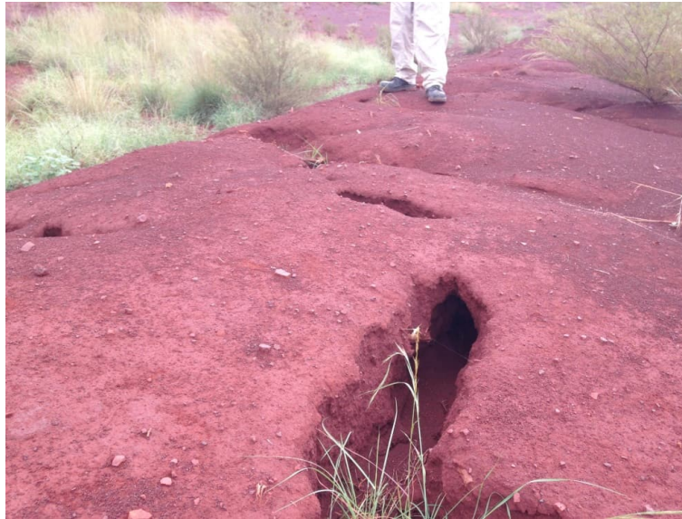
Too Fine (6 Years Old). Will need rebuilding
