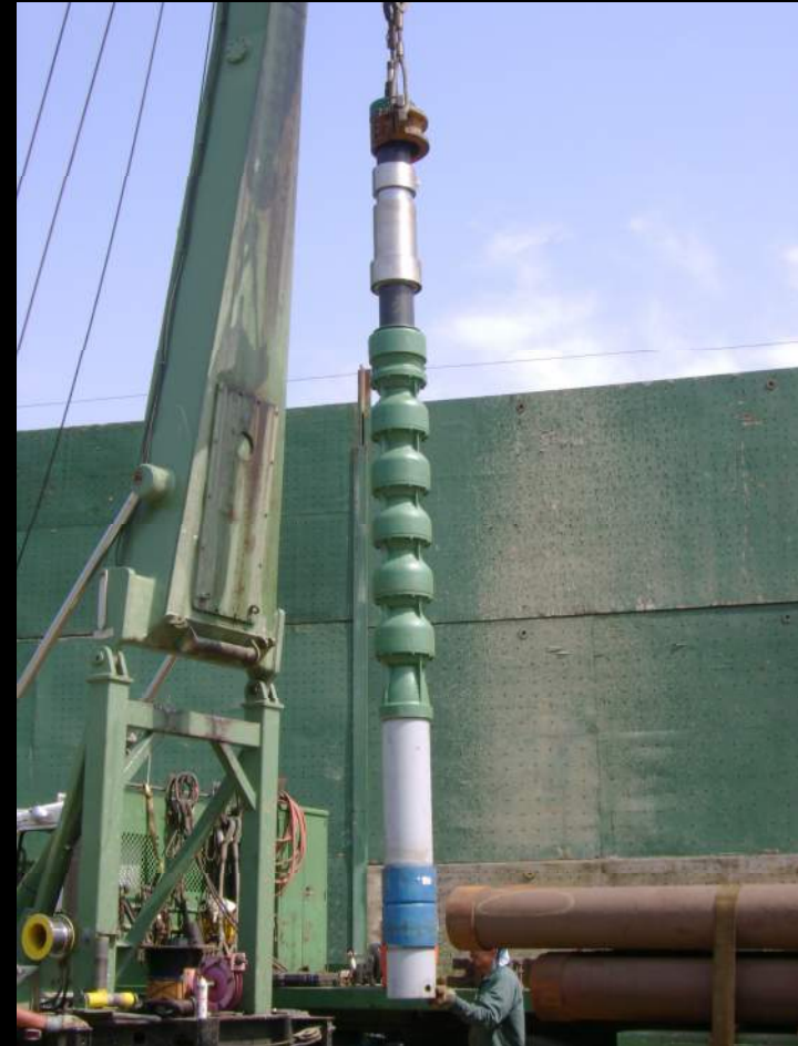
Installation of down hole flow control valve – Source R Tribble Cactus Controls
