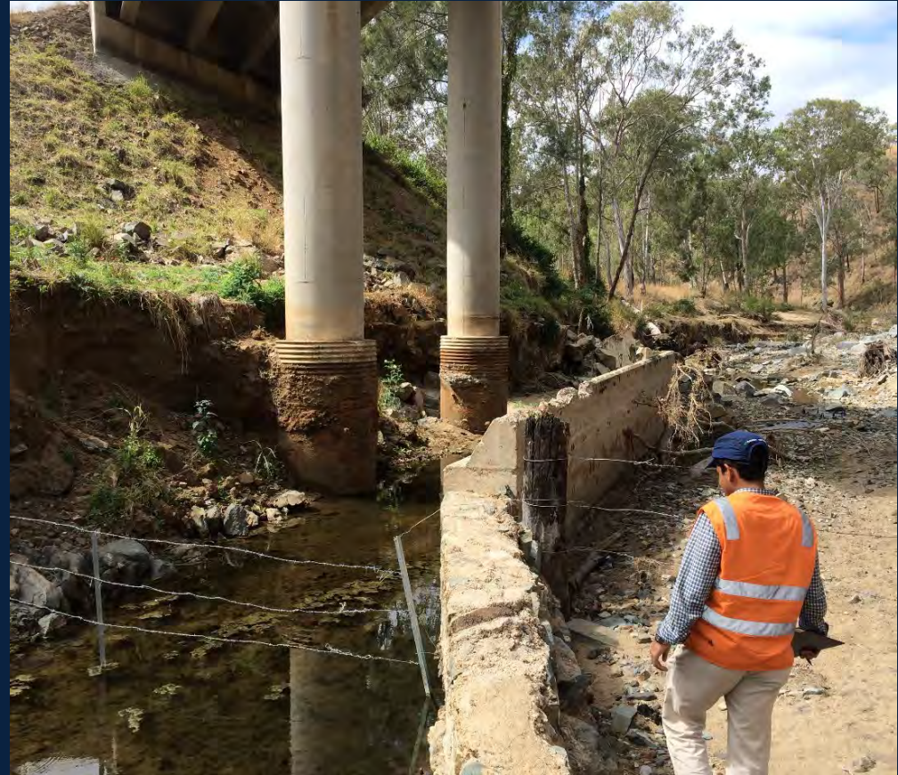
Collards Creek Bridge 5 after Cyclone Marcia, February 2015
