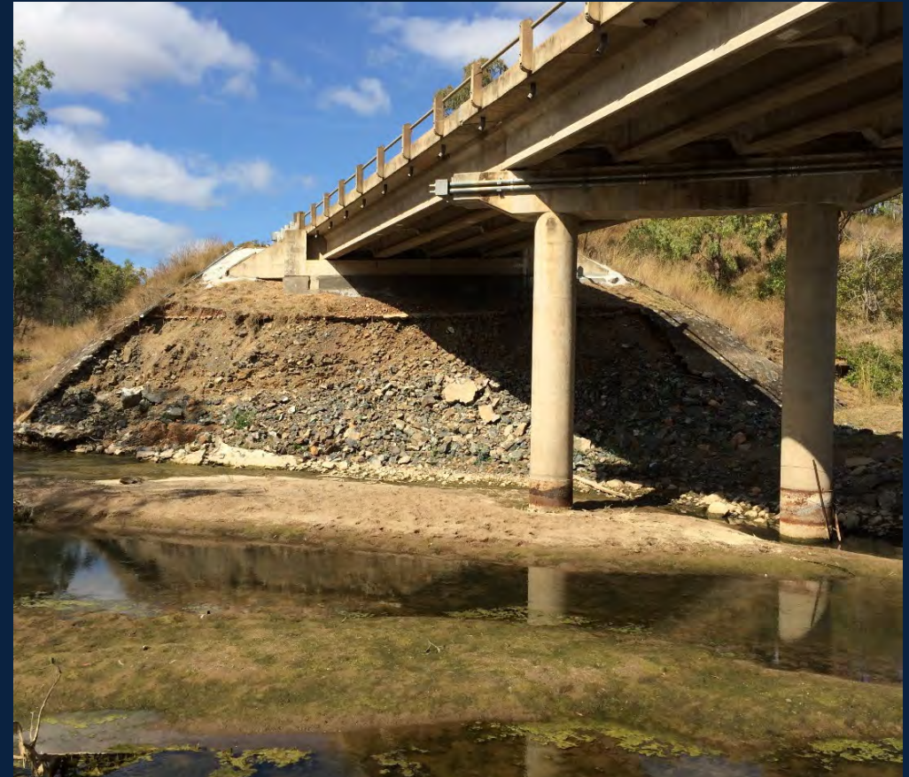
Collards Creek Bridge 2 after Cyclone Marcia, February 2015
