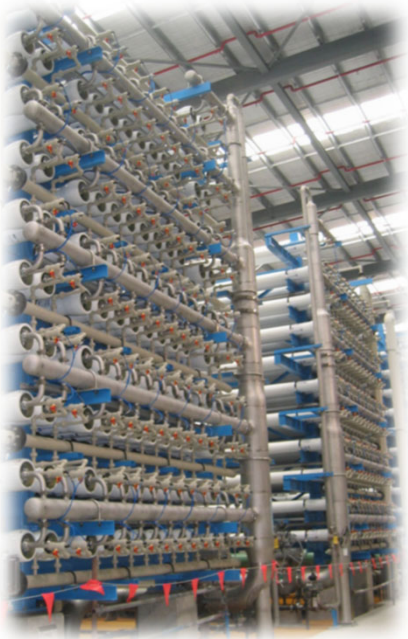
Vic Desal Plant Capacity 150 GL/y
